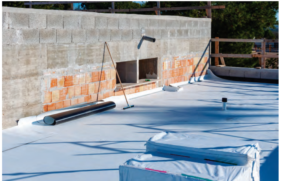
Roofs covered in thermoplastic polyolefin (TPO) can be significantly cooler than dark roofs when the weather is hot, greatly reducing energy demand.
