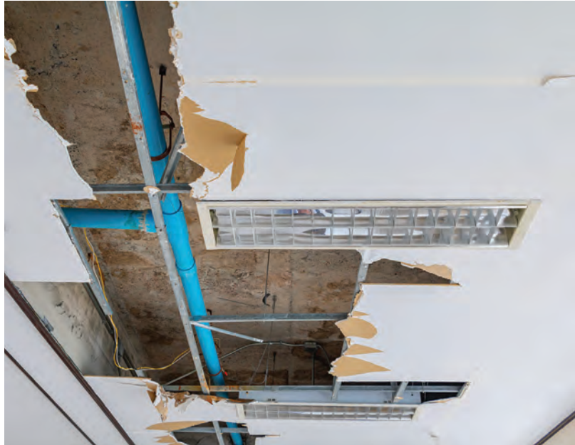
Plumbing systems are a major source of water damage and flooding in all kinds of commercial buildings.
