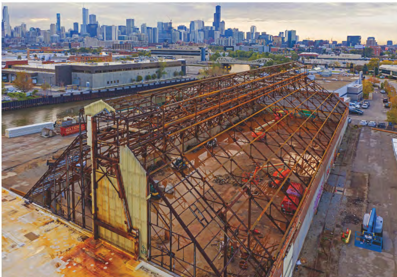
The metal framework of the salt shed. Preserving these trusses, which had been degraded by many years of exposure to salt, was one of the biggest challenges for the development team.
