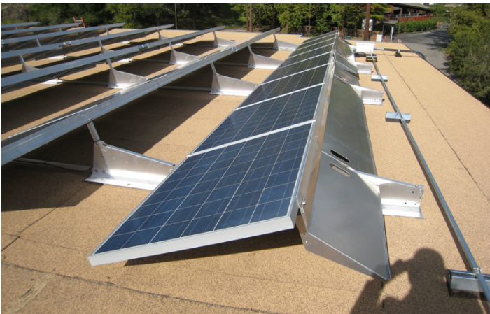
Rack-mounted array with masonry ballast blocks on an asphalt built-up roof. Note aluminum wind deflector at right. Image: Aaron Binkley
