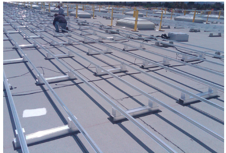
Field-assembled racking system under construction on an asphalt built-up roof. Image: Aaron Binkley
