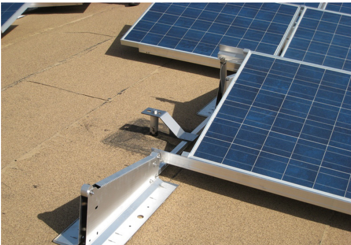
Solar racking permanently attached to roof structure. Note post with bolted connection. Image: Aaron Binkley
